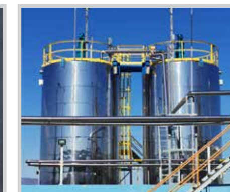
Sepro Mixing ammonium nitrate agitators
