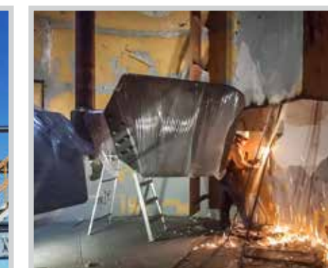
Sepro Mixing 11 1/2 ft (3500 mm dia) high solidity impeller installed
